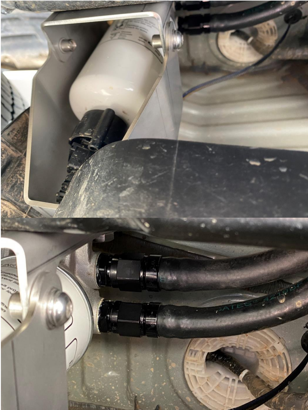
PreLine-Plus cover (LC300PL150.3) bolted in place
