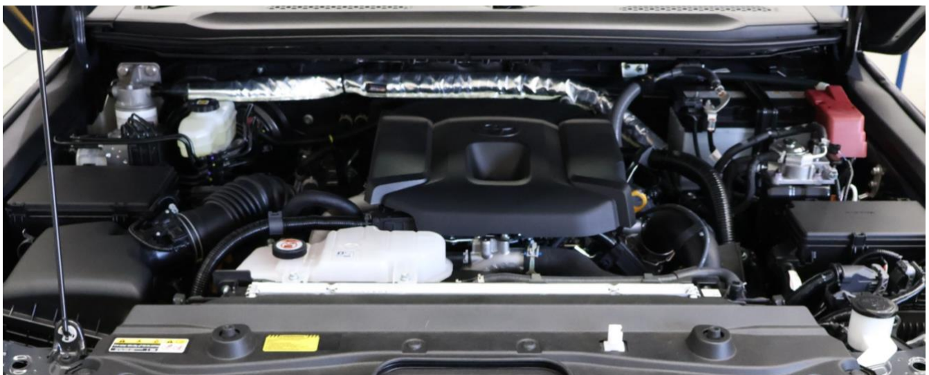
Finished installation showing hoses in place cable tied up across the back of the engine bay
